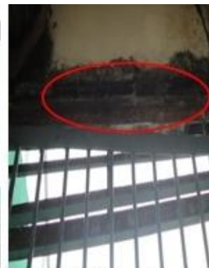
Photo=F4; Concrete spalling/ Rebars Exposed
