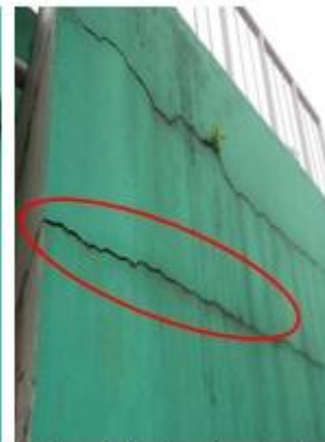
Photo= G2: Cracks seen in the walls.
