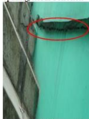
Photo=G1: Wall separation under beam
