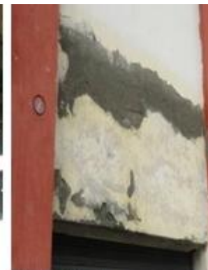
Photo=D1: Seepage Problem
