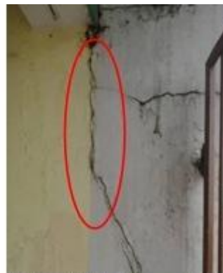
Photo=G3; Cracks seen at beam-column interface
