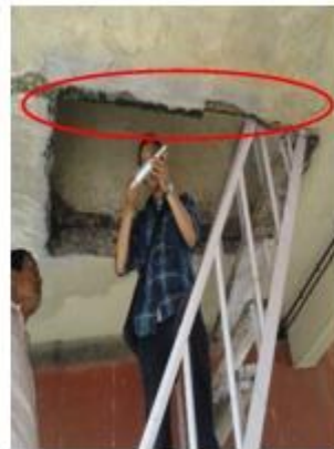
Photo=VIP 2: Concrete Spalling, Rebar Corrosion
