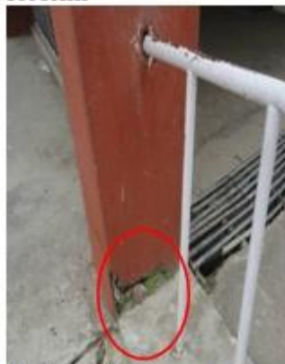
Photo=VIP4; Concrete spalling/ cracks seen
