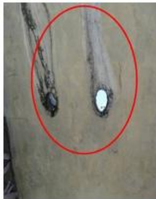
Photo=VIP1: Seepage Problem
