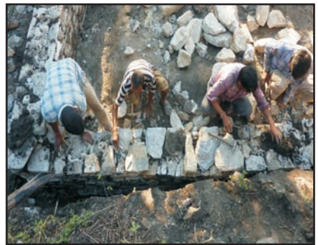
Looking at a wall from above the joint between the stones in the wall should not be in a straight line, but must be broken.
