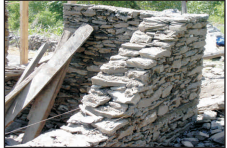
Construct all walls at the same time. If not possible then leave the wall end in stepped manner.
