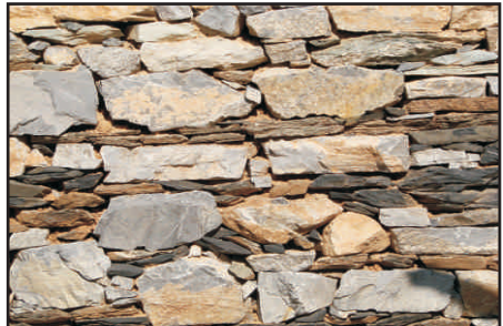
Each stone must be in contact with the stone under it, with little or no mud mortar in between.
