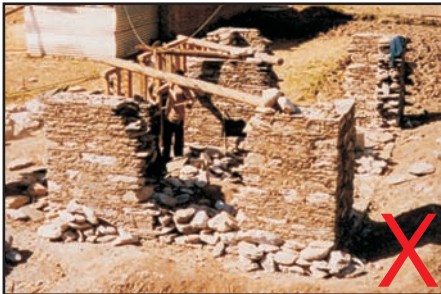
Never build corners first with tothing and then fill up the gaps between the corners. Construct corners and walls together.
