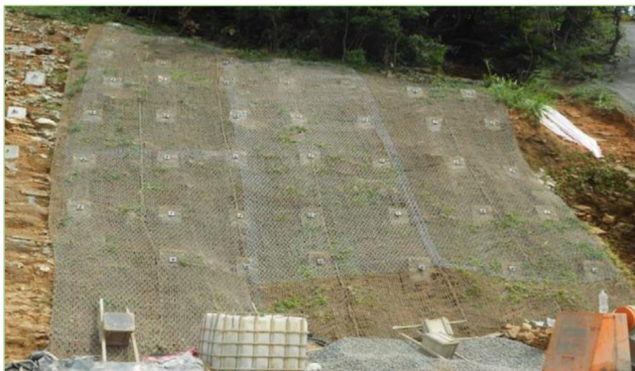
Figure 2-3 Nail heads connected by high tensile strength steel mesh and vegetation introduced by hydro-seeding with the help of coir mesh
