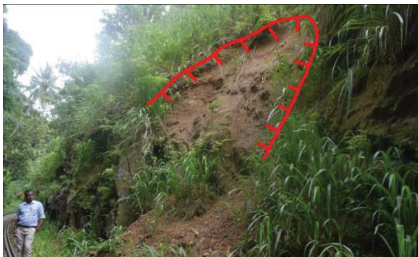
Figure 1-2 Failure of cut slope about 7 m in height in close proximity to the railway line in Ihalakotte – Balana (Mampitiyaarachchi, et al. , 2018)
