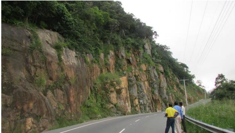
Figure 1-3 Location with rockfall threat. Kandy - Mahiyangana – Padiyathalawa road between culverts 55/3 and 55/6 (Source: http://nbro.gov.lk/ )
